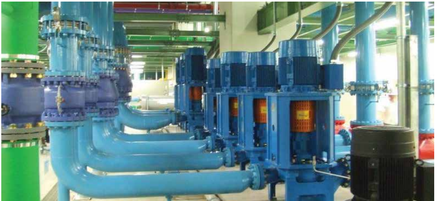
This ITT Goulds customer saved space as well as foundation and baseplates costs with seven Model 3910s. Many applications benefit from the inline piping as well.
