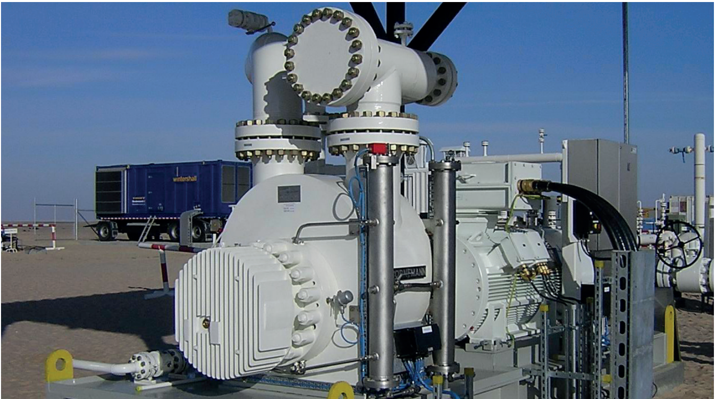
Multiphase „Boosting in Libya“
